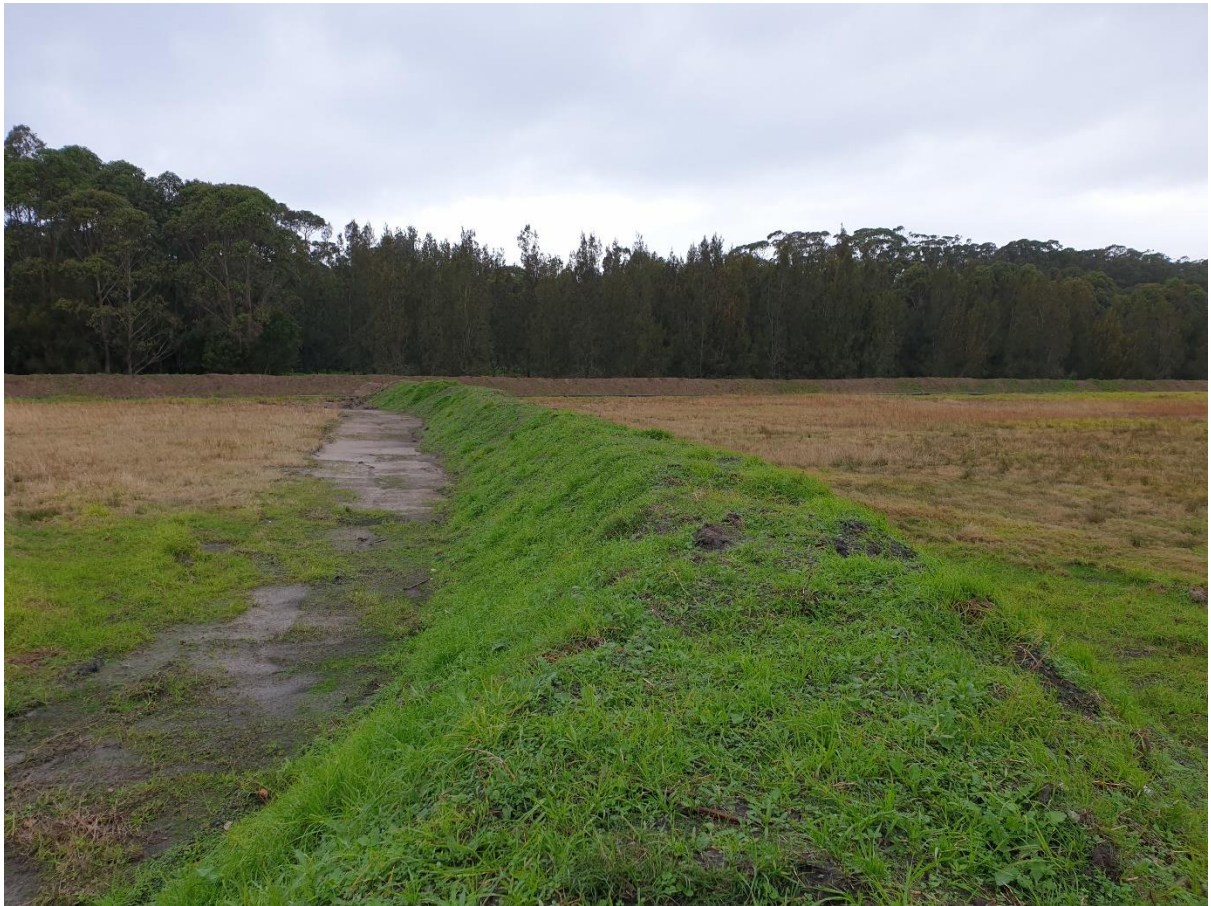
Figure 4 - Flood levees established in “CP” area (intermediate levee in foreground, boundary levee in background)
