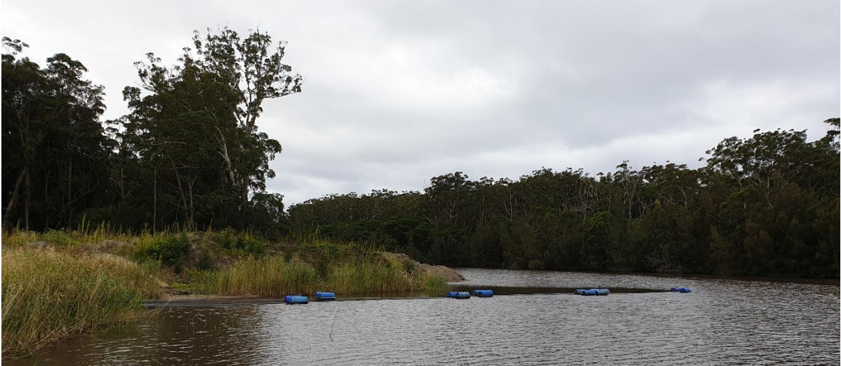
Figure 2 - Deepwater outlet on processing returns line running into the existing dredge pond
