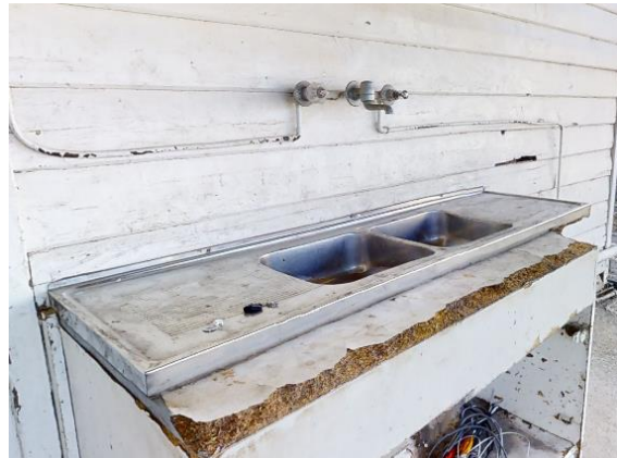
Figure 15: Laundry sink (Source: Cleary Bros. 3D Model – The ‘Belmont’)
