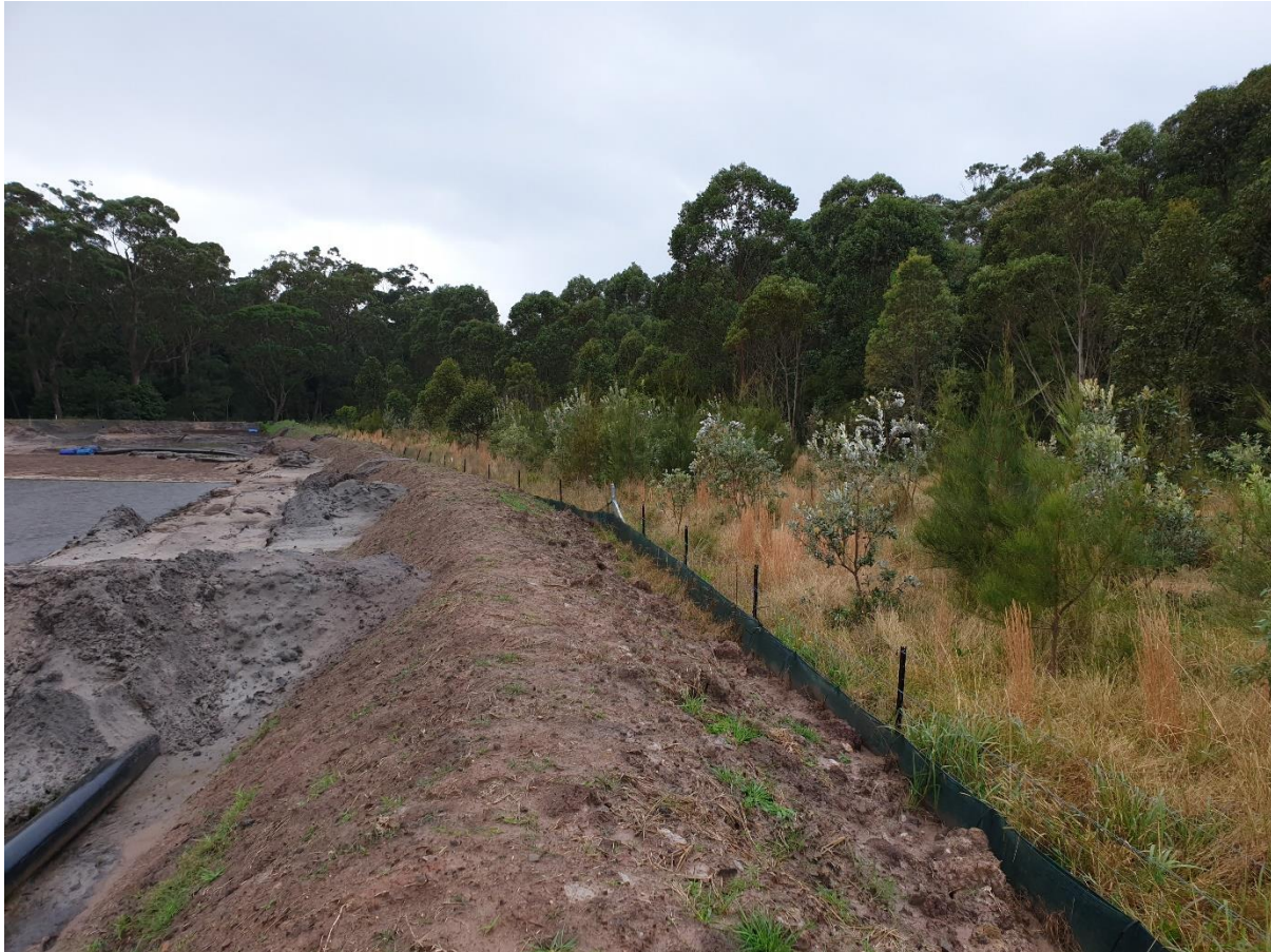
Figure 3 – Flood bund and sediment fence installed alongside perimeter of new dredge pond near zone 2C1
