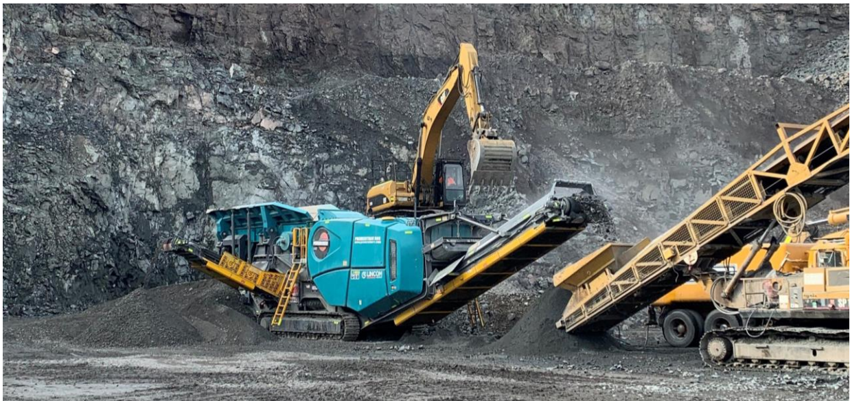
Plate 3.6 Premiertrak 600 Crusher and Screening plant being fed by an excavator (Ref: CB-3.4)
